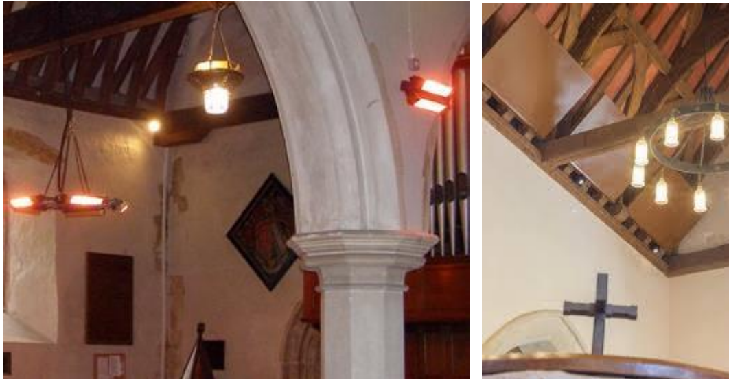
Figure 12: Left: Infrared radiant heaters installed at high level (SunSwitch) Right: Brown-painted radiant panels installed on ceiling (Solray)
