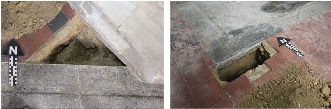
Fig. 7 Views of Test pit 3 (left) and Test pit 4 (right, showing ledger, limecrete screed and pier foundation, scale 0.15m
