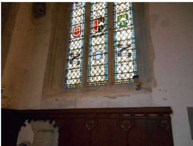
Damage to decorative finishes and wall plaster in Chancel (south side)
