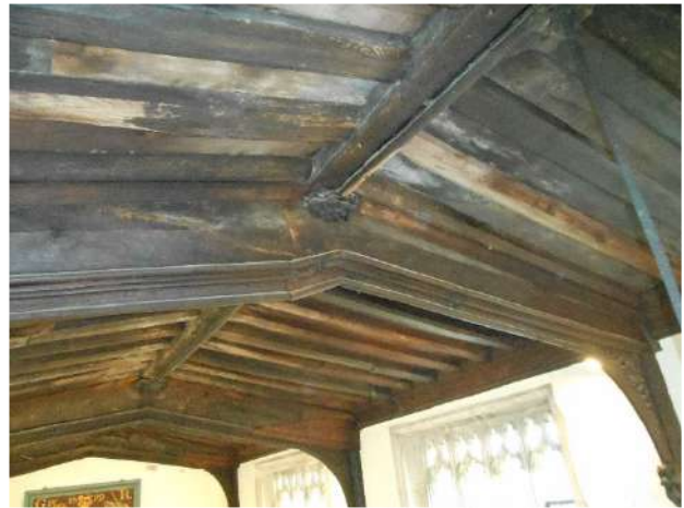
Staining (historic) to nave ceiling
