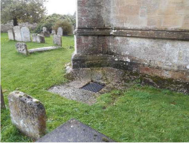
Moss becoming established and cracking/open joints to mortar flaunching and base of chancel east gable
