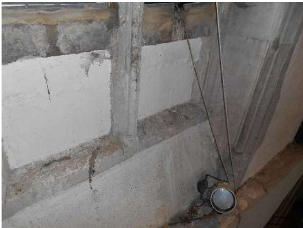
Example of water staining to painted panels below clerestory windows
