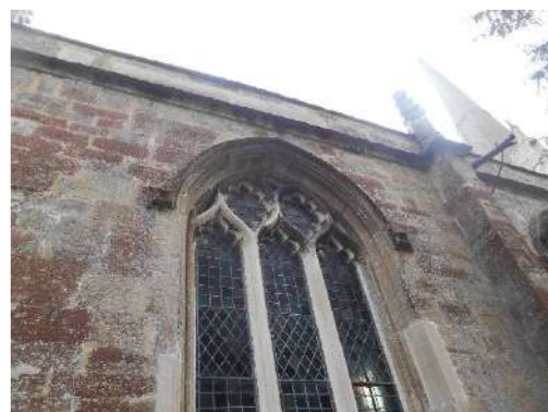
Potential open joints and displacement to hood moulding over north aisle window
