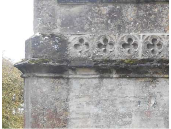
Pierced parapet block (lhs) to vestry north badly weathered
