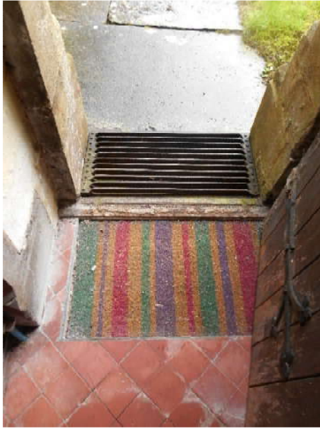
Corroding threshold to vestry external doorway
