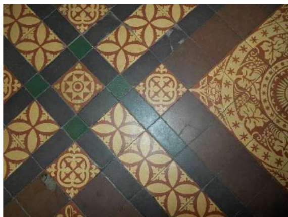
Broken/loose tiles chancel floor near sanctuary step
