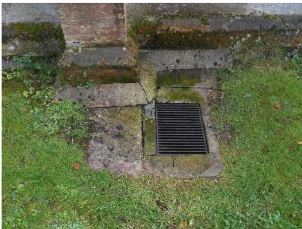
Example of open joints/cracking to aprons and flaunching's around drainage grates
