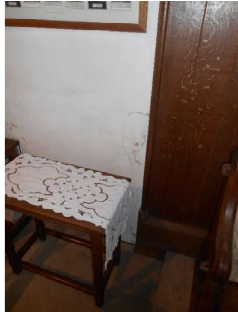
Damage to decorative finishes and wall plaster in Chancel (north side)
