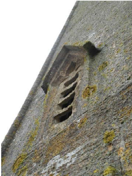
Example of weathering to spire lucarne louvres
