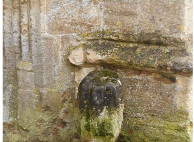
Spalling/localised loss of detailing to north porch plinth (nw buttress)
