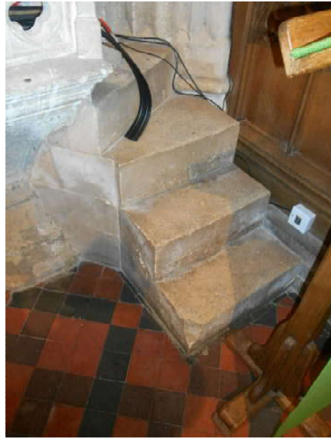
Damage (historic) to pulpit step
