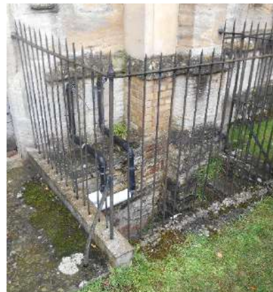
Corroding railings and gate around boiler room access steps
