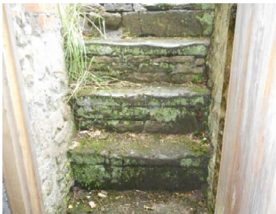
Vegetation, algae, debris and open joints to boiler room access steps
