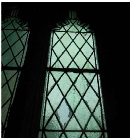
Damage to north porch window quarries (likely cause vandalism)
