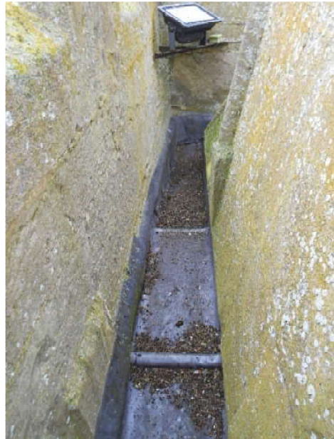
Debris build up to tower parapet gutter
