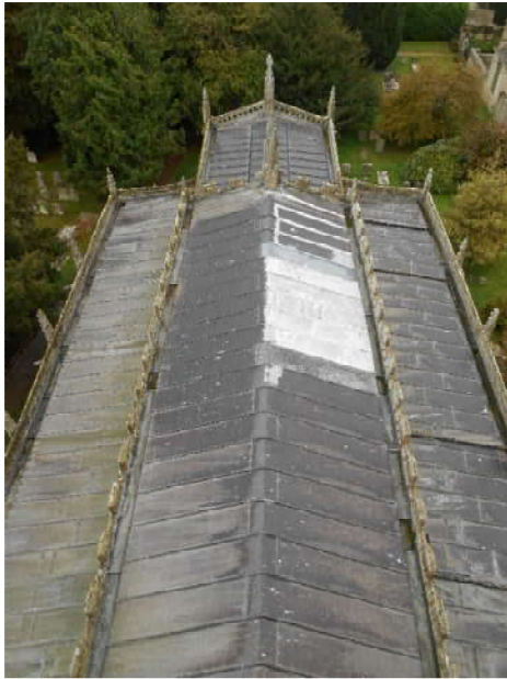
View looking east from tower parapet, across lower roofs of nave, chancel, north aisle and south aisle
