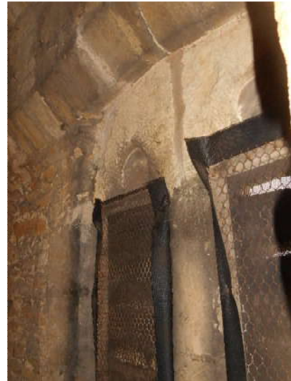
Corroding chicken wire covers to inside face of belfry louvres (to stop birds accessing the space)
