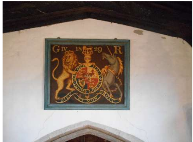
Failed decorations to nave east gable and cracking in plaster above chancel arch stone detailing
