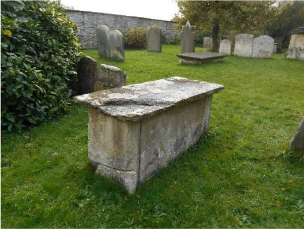
Example of condition of some chest tombs in churchyard (photo south side of churchyard)
