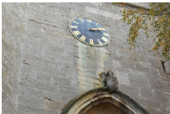
Staining below tower clock face
