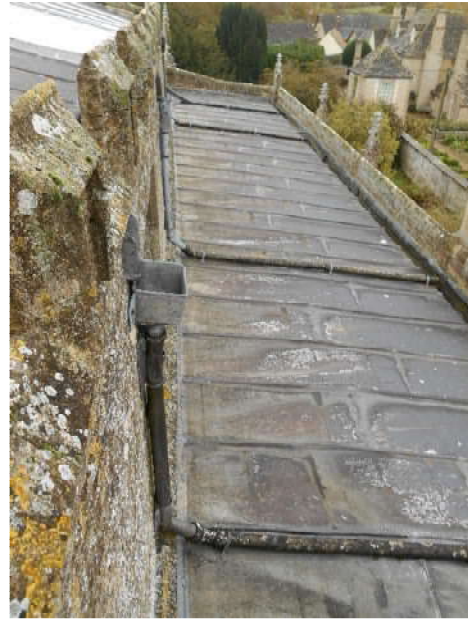
View across south aisle roof (from nave) looking east, with asbestos pipework transferring rainwater over roof and shadowing of sarking boards below clearly evident
