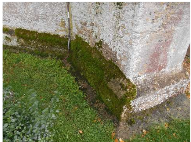
Example of moss growth to external wall plinths (photo – northwest tower buttress)
