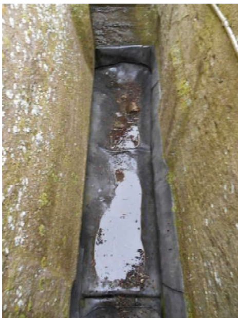
Water pooling to uneven bays to tower parapet gutter
