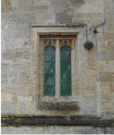
Partial loss of hood mould and stop to north porch west window
