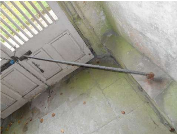
Algal staining to floor and lower wall areas of north porch – as well as failures/wear to decorative finishes
