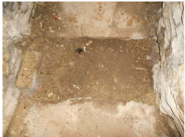
Dampness to floor
