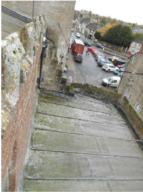
Stone steps from nave roof to north aisle (west) roof – open sided with single handrail only and no other safe safety measures over sheer drop
