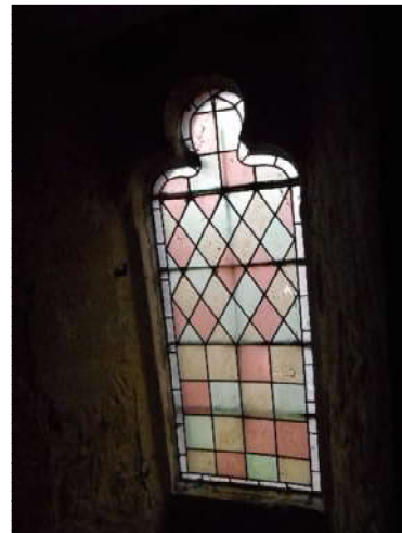
Damage to clock chamber window
