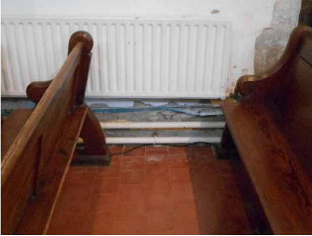
Example of plaster damage to base of south wall to south aisle
