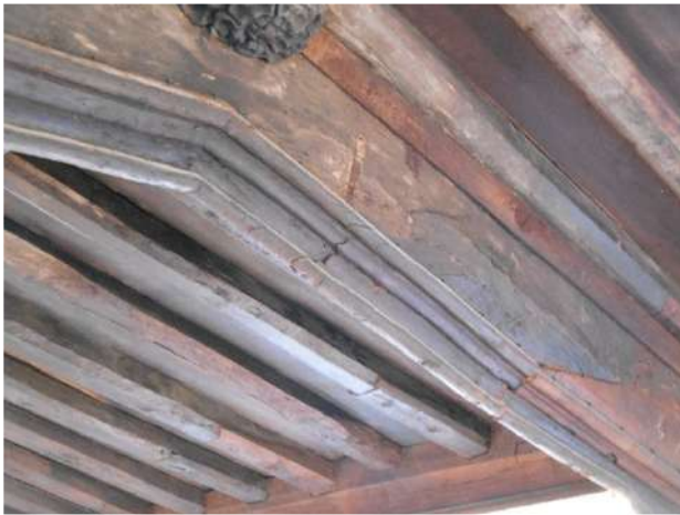
Previous repairs to nave ceiling
