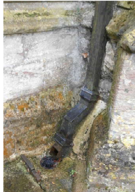
Staining and surface corrosion to base of North Aisle/Vestry downpipe
