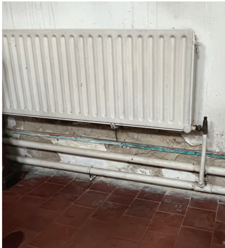
▲ The damaged walls and old heating system ▲
